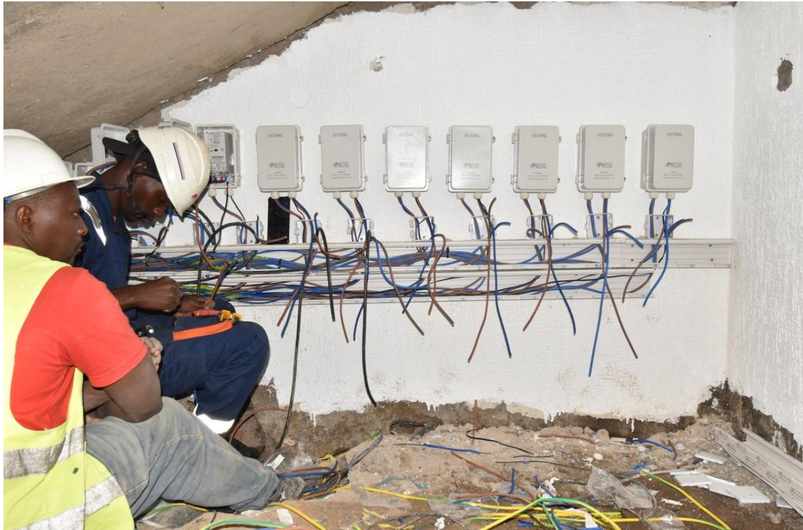
REC connecting cash power for phase 1
