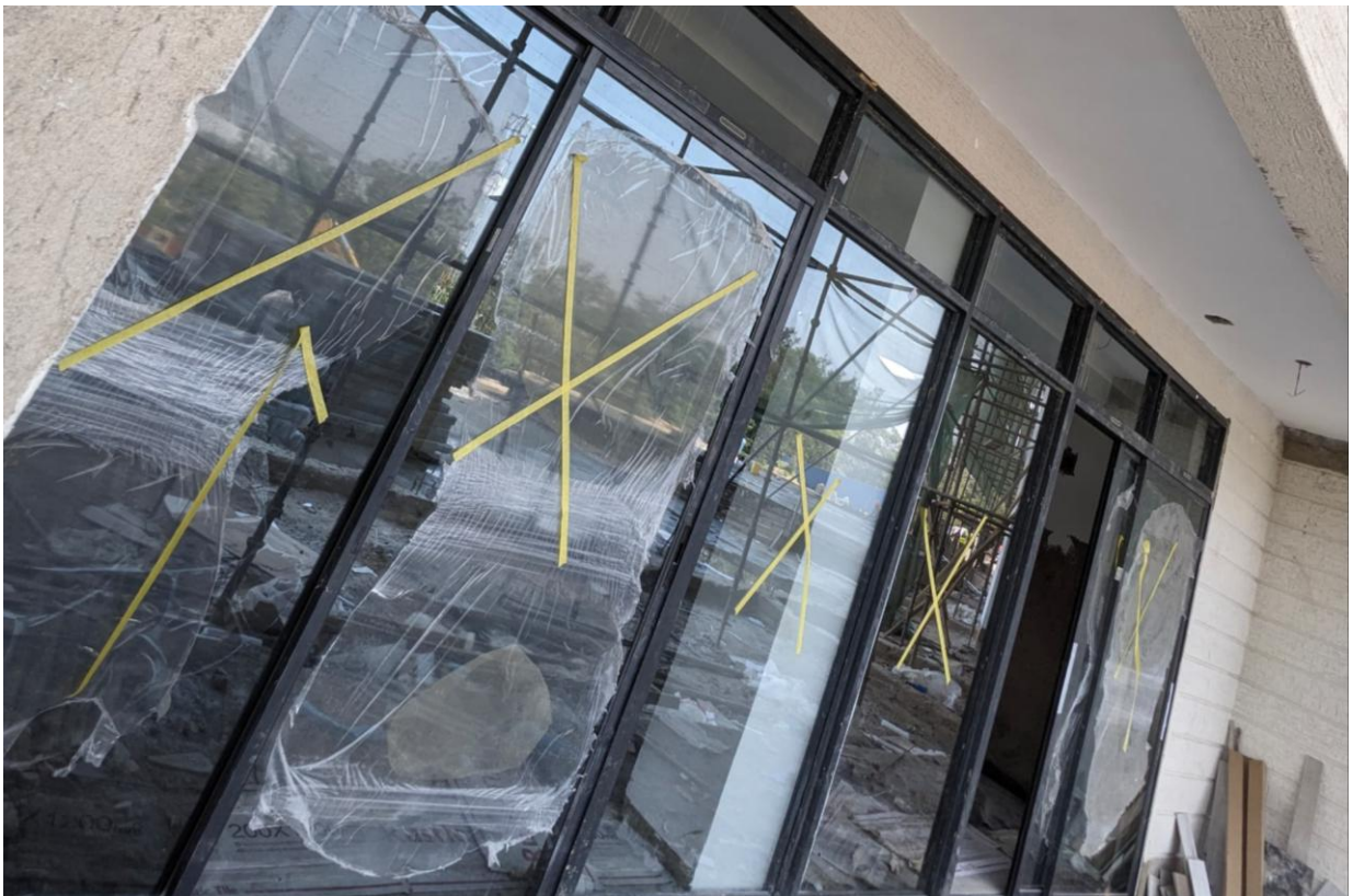
Phase 2 works showing: Curtain wall glazing installed in one of the units
