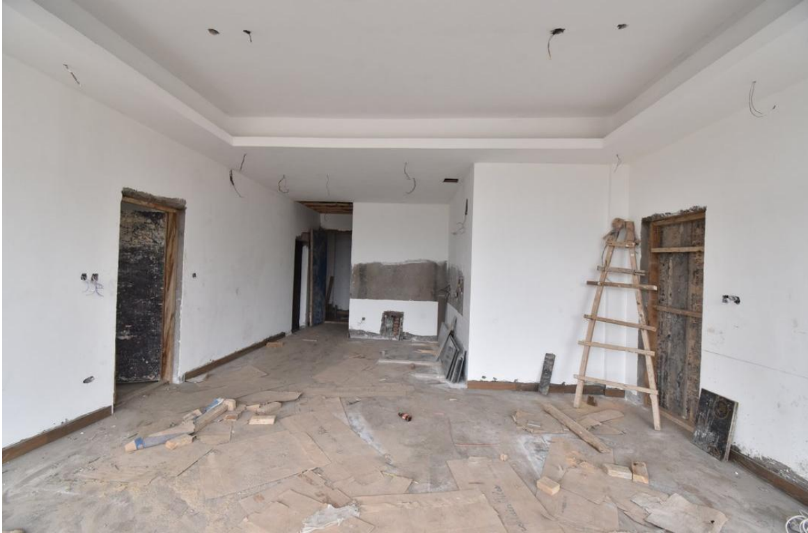
One of the units Phase 2 showing tiles done, gypsum and first coat of paint
