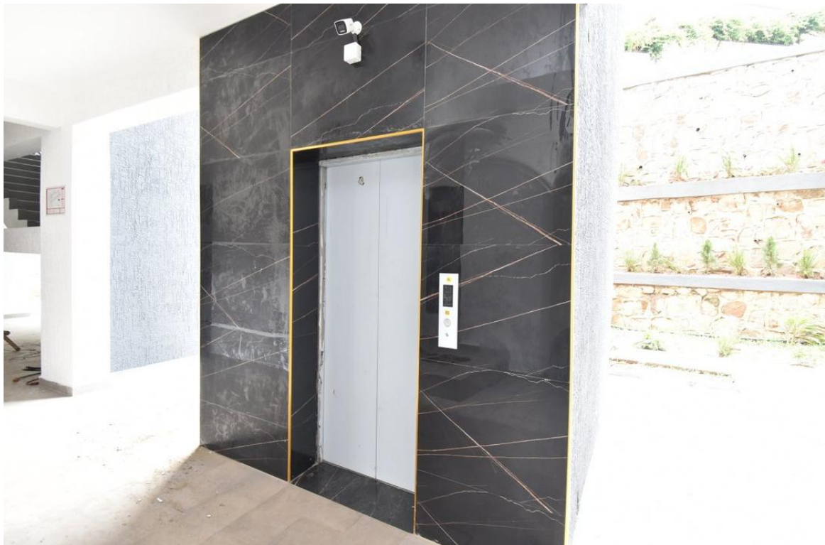
Lift at Phase 1
