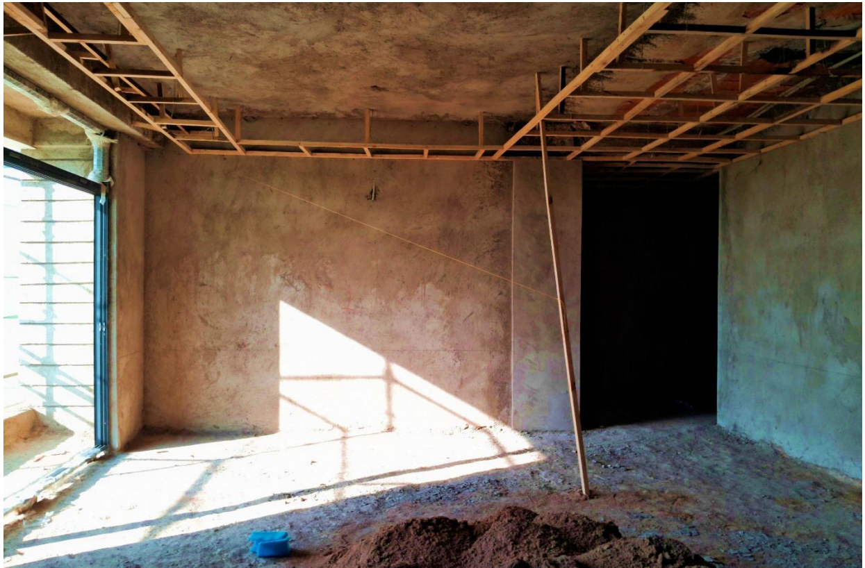
Phase 2 works showing: Internal plaster and ceiling work in one of the units
