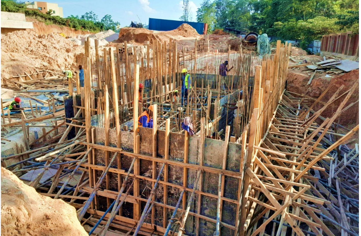
Phase 2 works showing: Steel reinforcement and formwork for Lv. 2 walls of wastewater treatment plant
