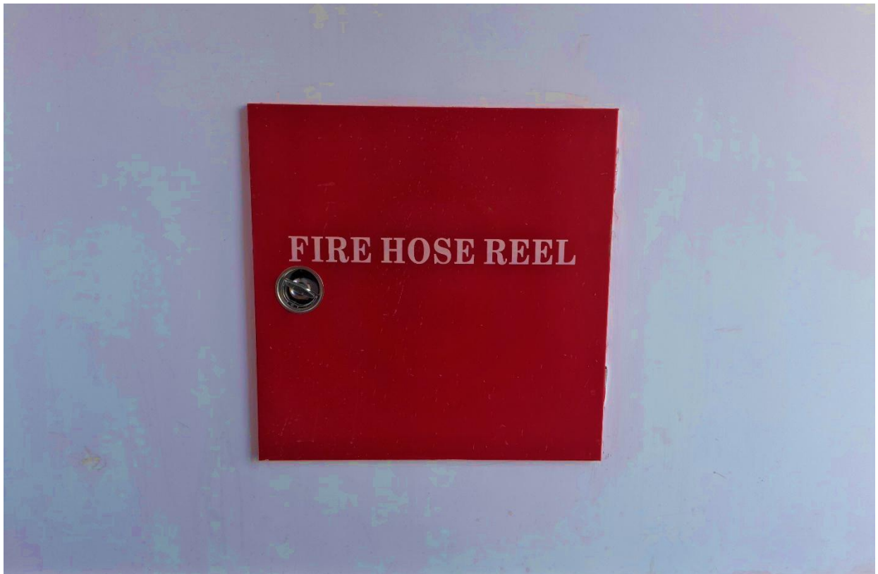
Phase 1 works showing: Fire hose installations in place
