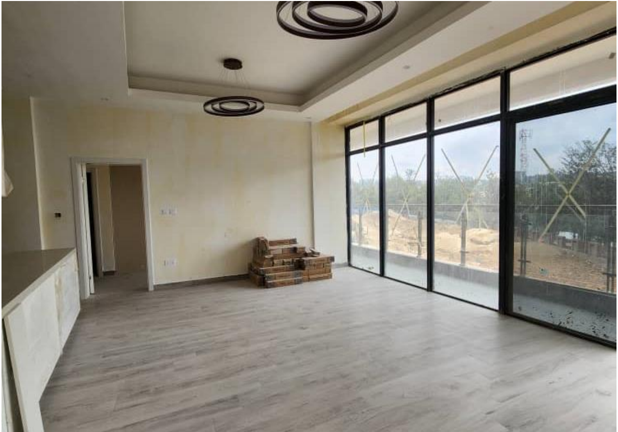
Phase 1 showing one of the units, ready for painting, power installed and working
