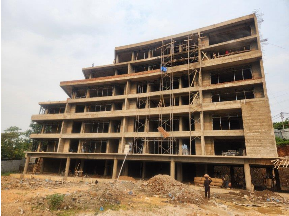
Front View of on Phase 1
